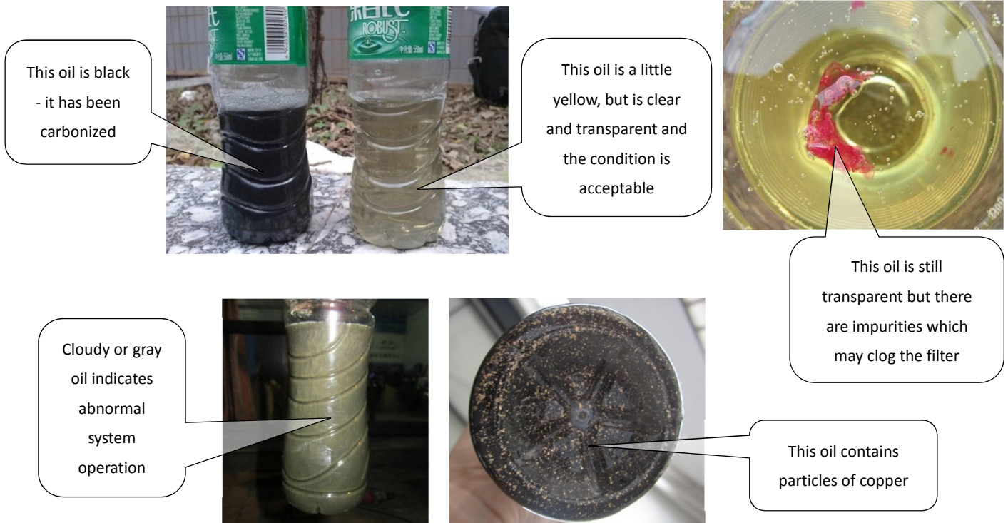
Figure 4-4.11: Inspecting compressor oil
