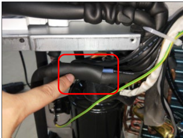
⑥Return air pipe temperature sensor
